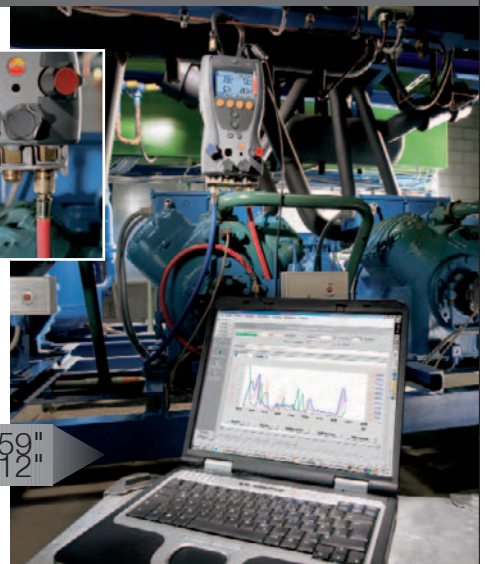
Service and maintenance on a refrigeration system using testo 556 and 560, commissioning included
