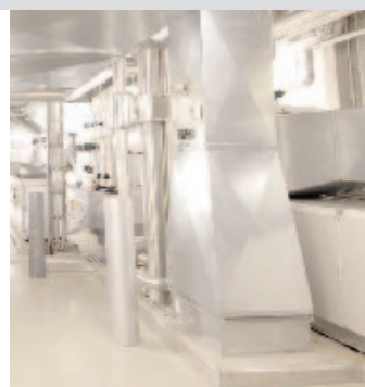
Monitoring ambient conditions in ducts
