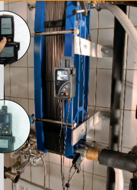
Checking technical systems (flow/return temperature) in production facilities
